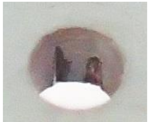
Insertion depth too low
